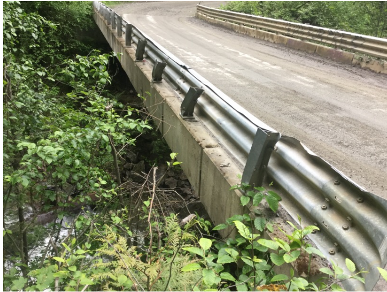
Damaged guardrail and risers entire upstream
