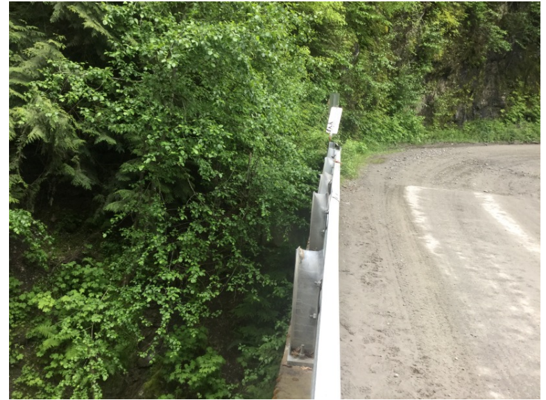
Upstream guardrail damage
