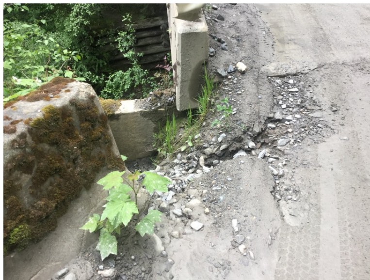
Fill erosion down stream left bank
